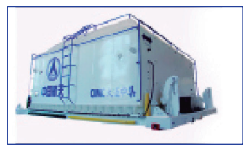
Generator / Voltage Transformer Container
