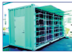
Energy Storage Peaking Power Station
