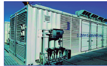
Energy Storage Peaking Power Station
